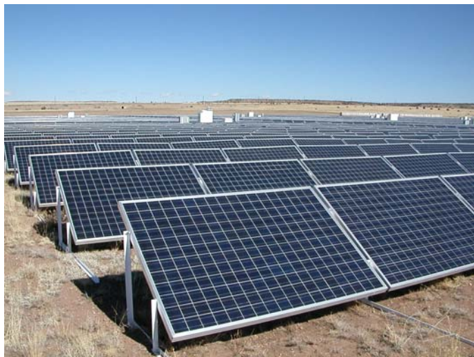
Figure 2. Typical 135 kWdc System
