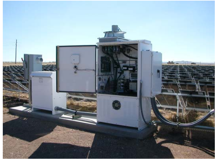
Figure 3. Xantrex PV-150 System Inverter
